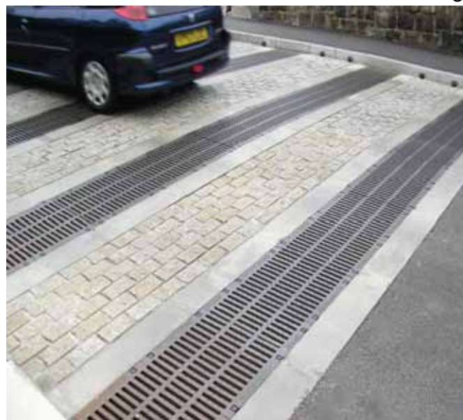
FASERFIX® fibre reinforced concrete channels with ductile iron gratings installed at St Ives, Cornwall as part of a flash flood prevention scheme
