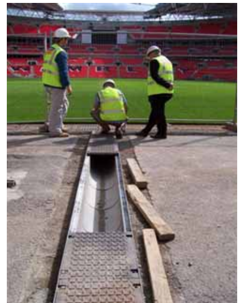
Hauraton cable management channels featuring SIDELOCK® ductile iron covers being installed in a major UK stadium
