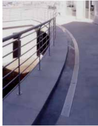
DACHFIX® drainage channel on a walkway
