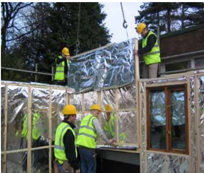
Eco-Brite in pre-fabricated cabin walls
